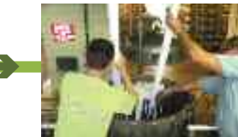
Raw water at the West Water Plant is pretreated by cartridge filters to remove particulates
